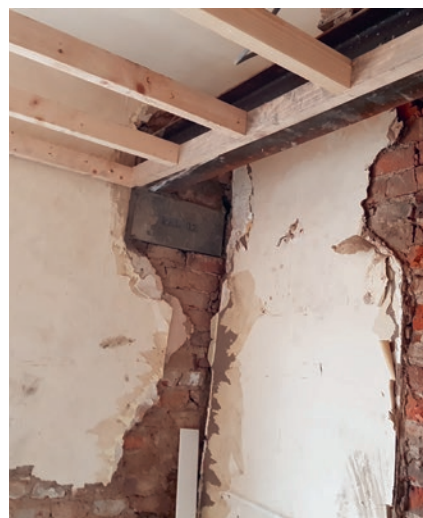
1. Example of L-section beam in place and alternative angle of defect
