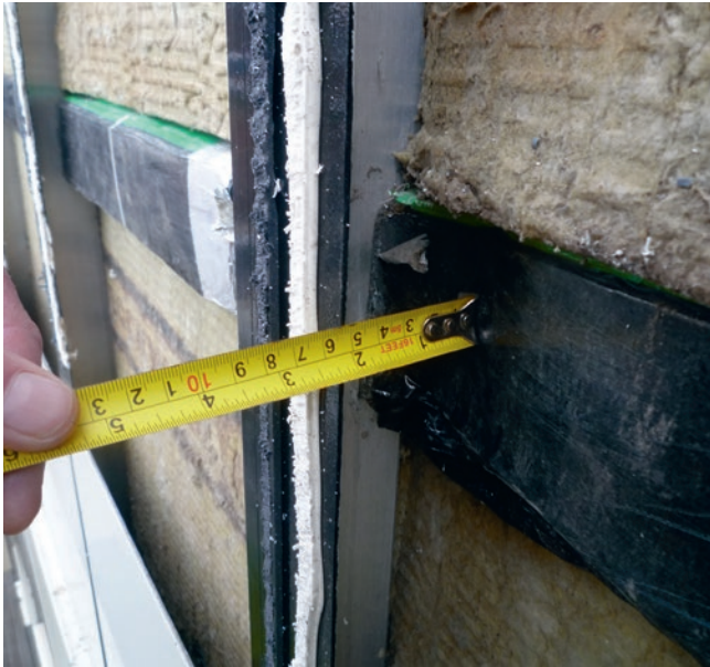
Indifferent and excessive installation of cavity barriers
