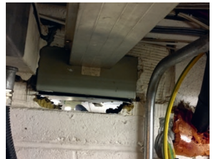
Disturbed fire battery compartmentation
