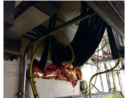
Poorly applied expanding foam repair
