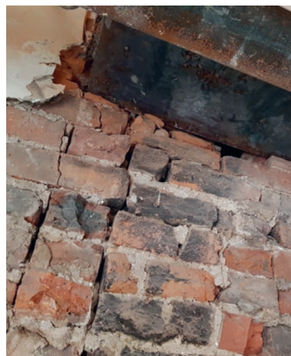
2. Damage to party wall by chimney removal
